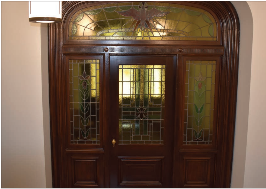
The original entrance doors, encased in the front entrance, and staircase remain intact.
